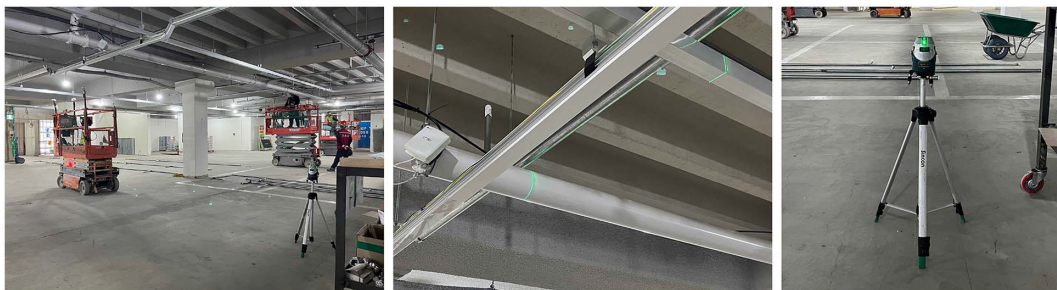
Fig. 1. Alignment of plumbing using a 360° line laser level in a basement construction site. Image courtesy of Hyundai E&C. (Images by Sungbo Yoon.)
