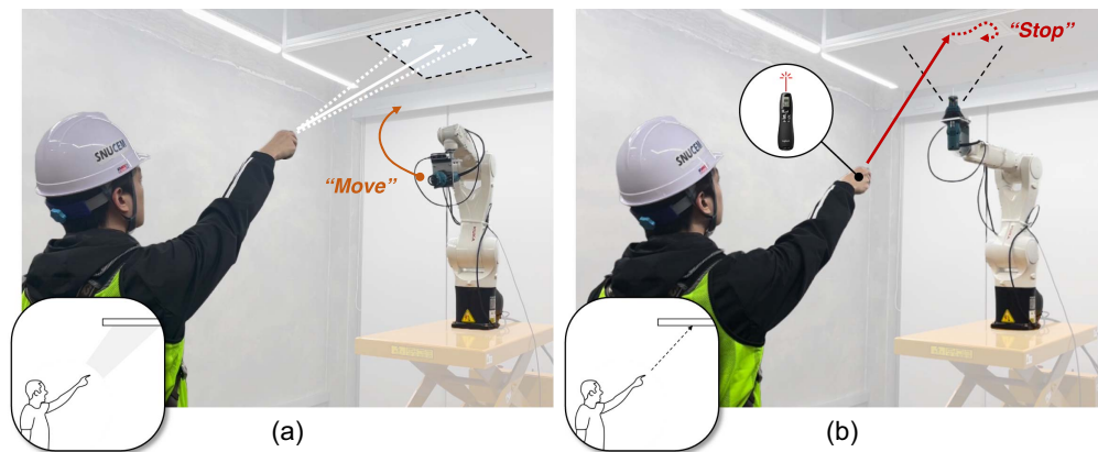
Fig. 2. Proposed global-to-local identification approach for spatial tasking in a drywall cutting scenario: (a) global guidance to indicate the general area; and (b) local refinement to precisely specify the cutout shape. (Images by Sungboon Yoon.)
